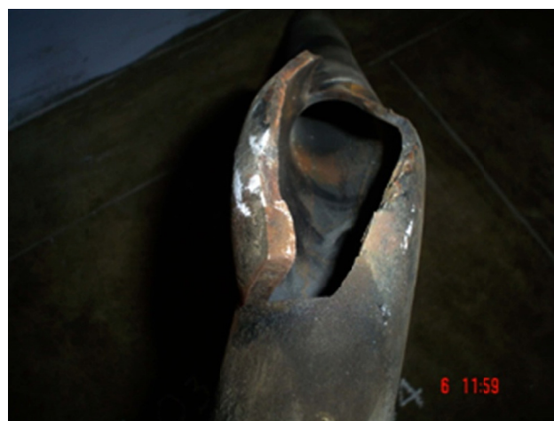
Fig. 1. Failure in inlet pigtail pipe bend
