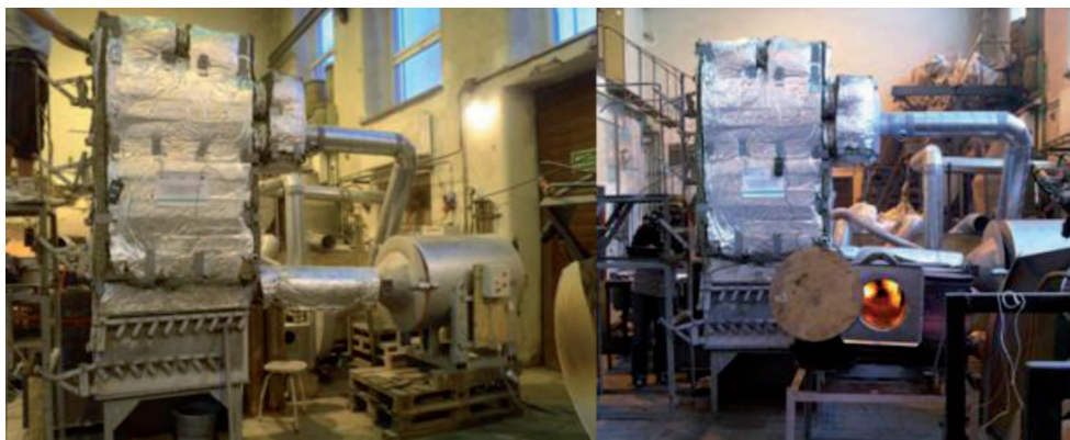
Fig. 6. View of the new dryer
